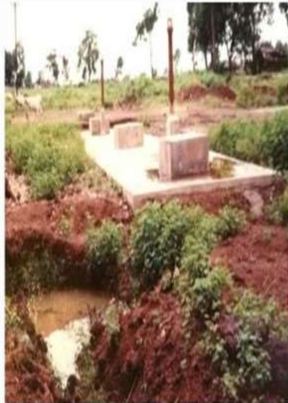
Overflowing Soak Pit due to impervious soil
