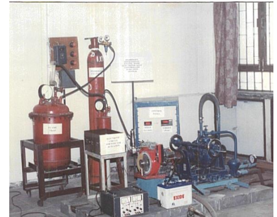
Neat Hydrogen-fuelled S.I. Engine Genset
